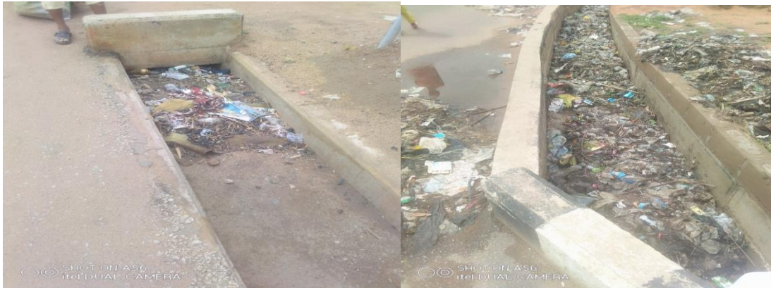
Plate 3. Showing the Improper dumping of waste in gutters/culverts along Abuja Road in the study area captured on June, 2022.
